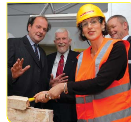
Lincoln MP and Public Health Minister Gillian Merron starting the refurbishment work at the Homer House 'wall-breaking ceremony'
